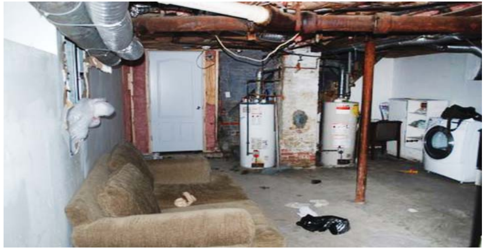
Illegal units, such as this one found in an apartment building basement, put all building tenants at risk.
