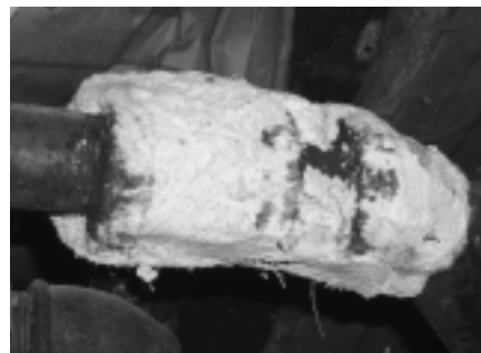
Asbestos used as pipe covering.
