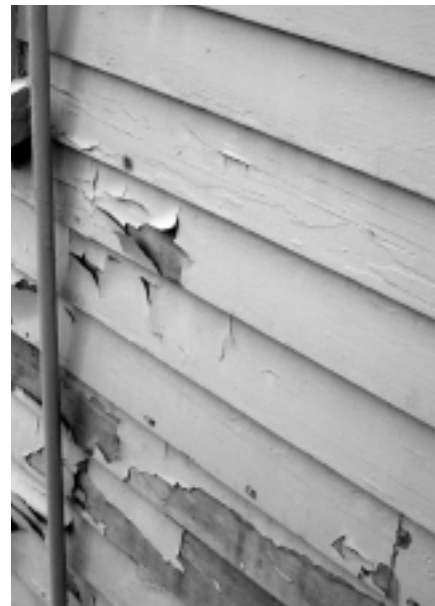
One thing inspectors will check is that the exterior of the building is weather resistant and that no paint is peeling and siding is not exposed to the elements.
